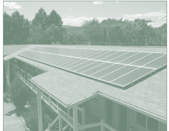
The Thunder River Lodge 10.64 kW solar
