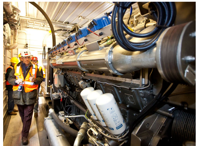
One of the methane plant generators
