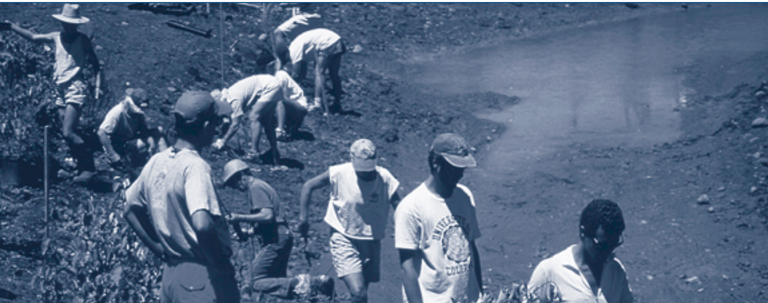
Construction of the Marolt Wetlands, a project funded by the Environment Foundation.
